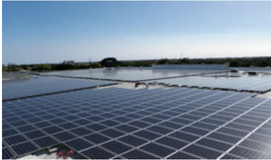
2.5 MW Navy PV Rooftop Systems (Largest PV Array in Hawaii)
